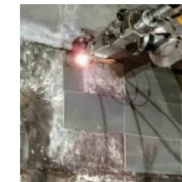
Anti-cavitation coating on hydro power station
